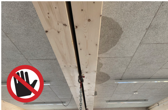
Leaky module joint
