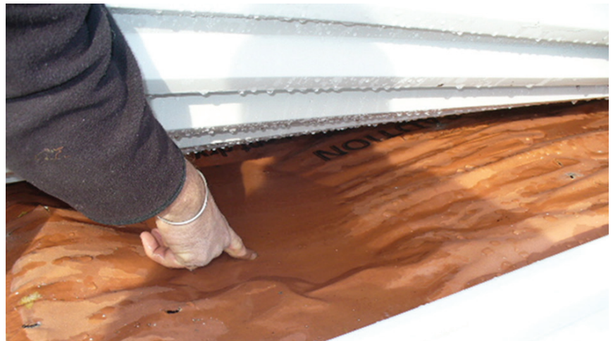
Figure 9. Ponding of a membrane installed in NZ at extremely low pitch with no rigid support board or structured ventilation strategy.
