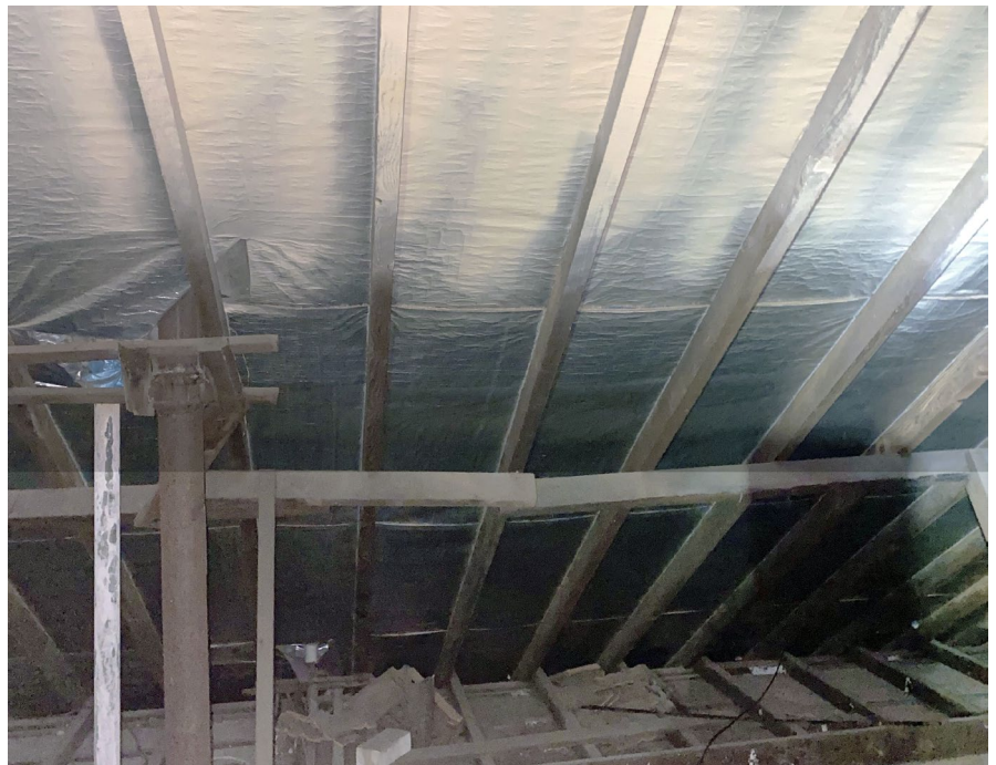
Figure 4: Foil has become engrained in the psyche of the Australian building industry as a one-sided solution to improve summer performance of buildings. But installing a vapour barrier, such as foil, can lead to perverse outcomes during winter. (Image: Sean Maxwell)
