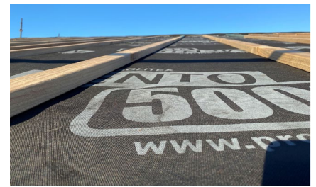
Figure 13: With purpose-built cavity the counter battens define the ventilation cross-sectional area. The type of cladding, metal or tiles is therefore irrelevant and only changes the batten spacing. (Image: Pro Clima Australia)
